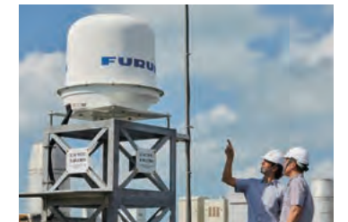
(Compact Weather Radar installed at PUB, Singapore)
