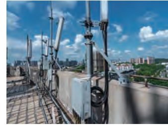
(5G Mobile Base Station)
