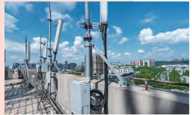
5G mobile base station
