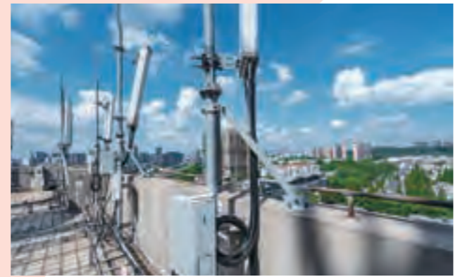
5G mobile base station
